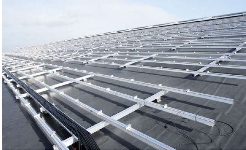
Aluminum racking fastened through roof deck
