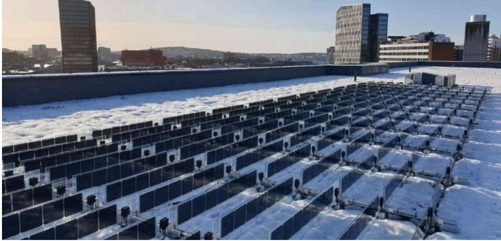
Vertical Bi-Facial Installation Switzerland, Photo Courtesy of Over Easy Solar
