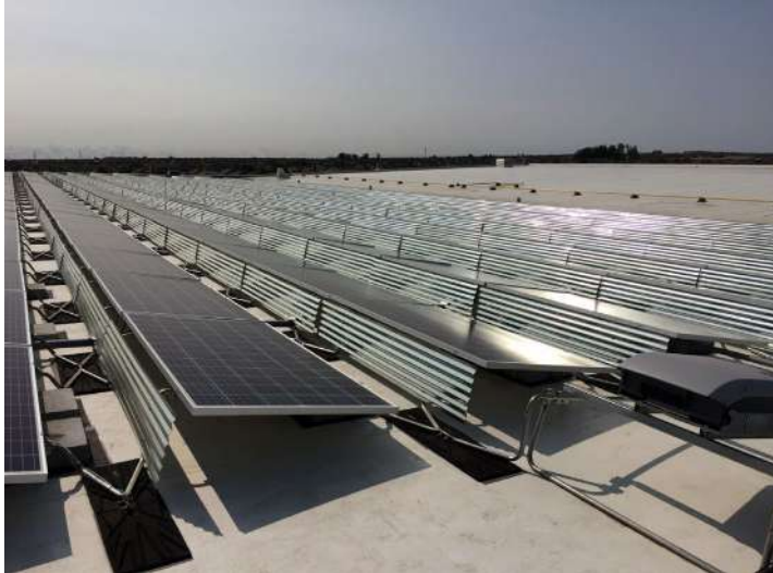
Non-penetrative ballast system on roof.
