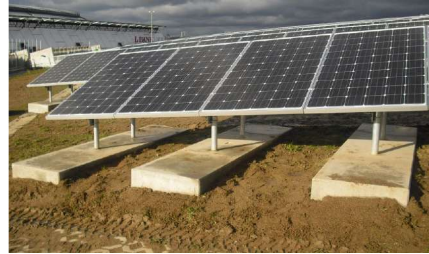
Ground mounted system on concrete foundations
