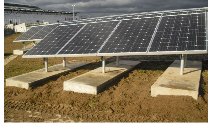
Ground mounted system on concrete foundations
