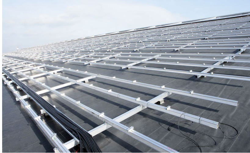
Aluminum racking fastened through roof deck
