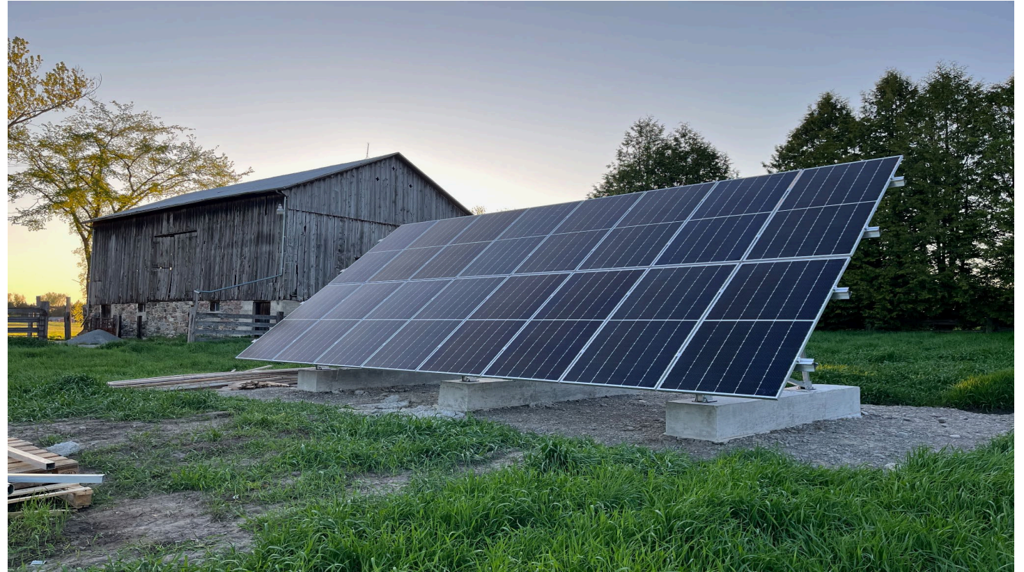
Photo Courtesy of Sponge Microgrids Inc.
