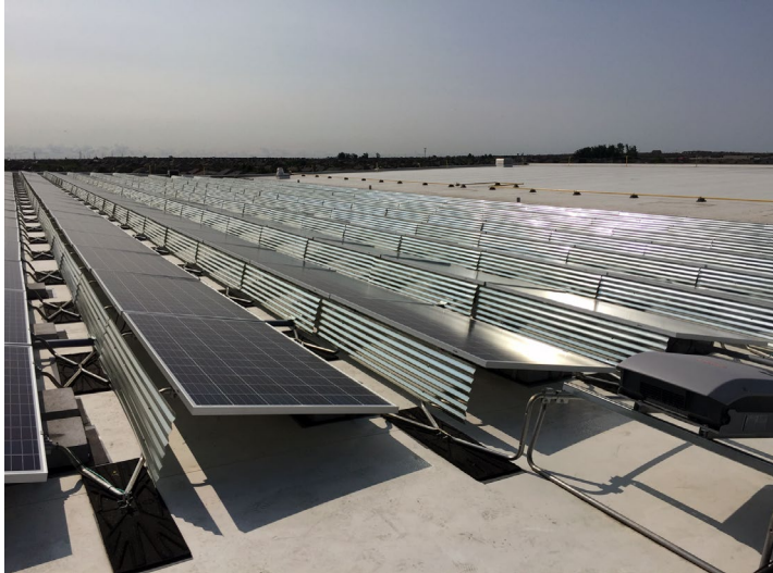
Non-penetrative ballast system on roof.
